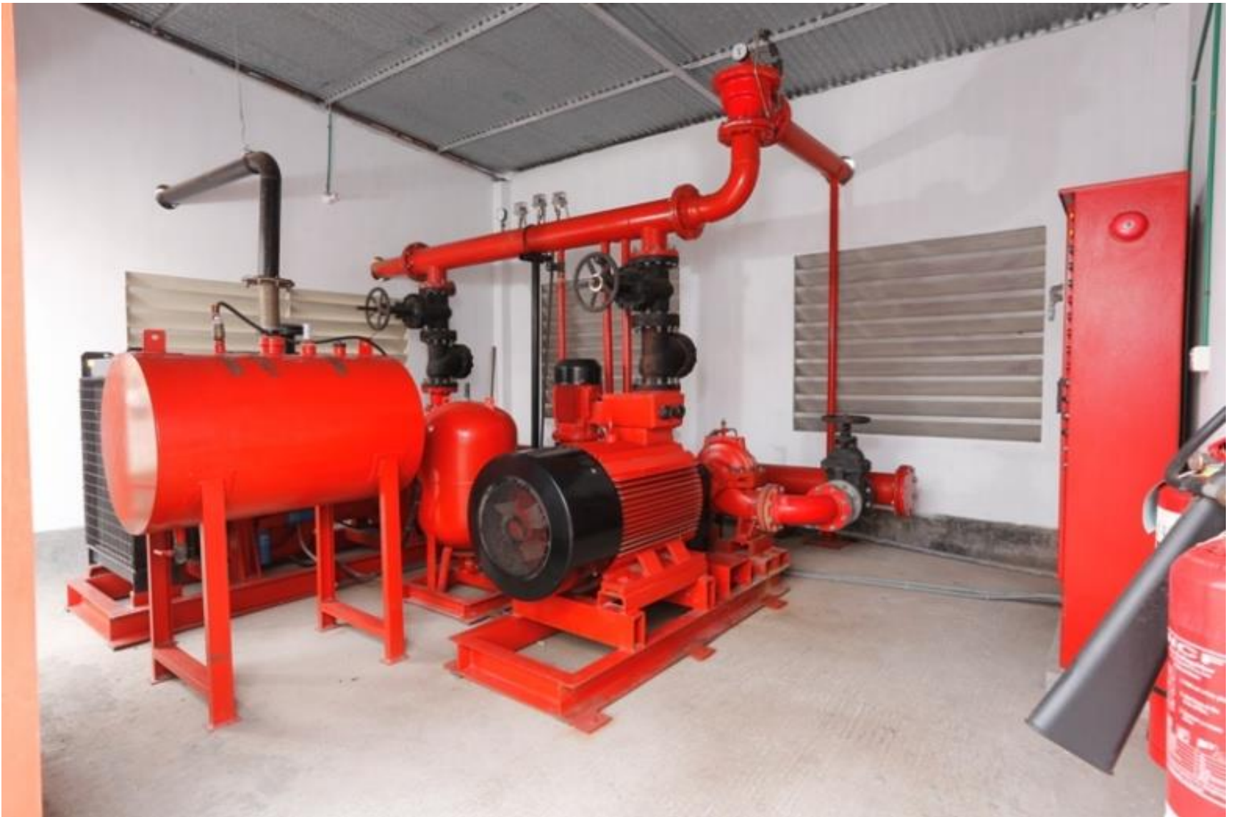
Central Fire Fighting system
