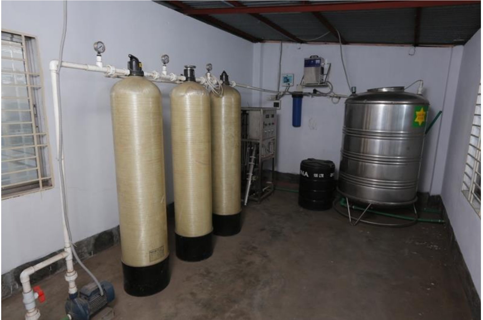
Drinking water purification system
